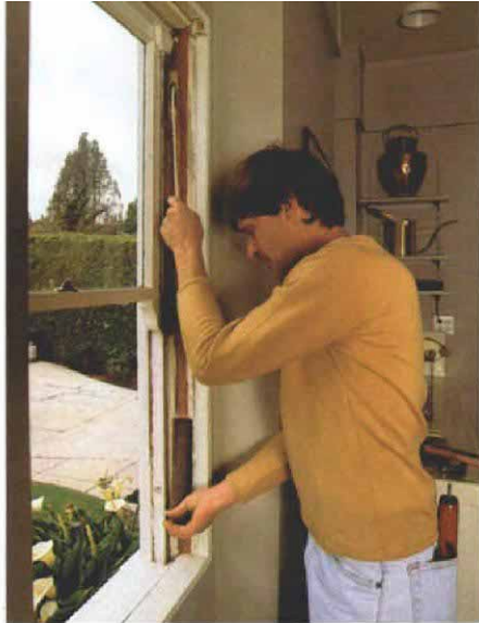
To retrieve the sash weights, the author cut access holes in the window frames. When reassembled, the hole will be plugged and almost completely obscured by the interior stop. Here Strawderman reinserts a sash weight into its chase after attaching a new cord to it.
